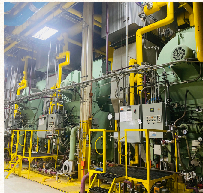
New steam boilers in one of the Central Utility Plants
